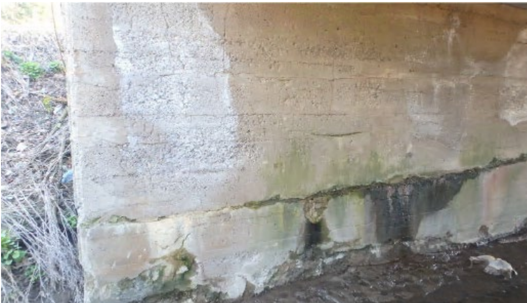
Spalling and deterioration at cold joint
