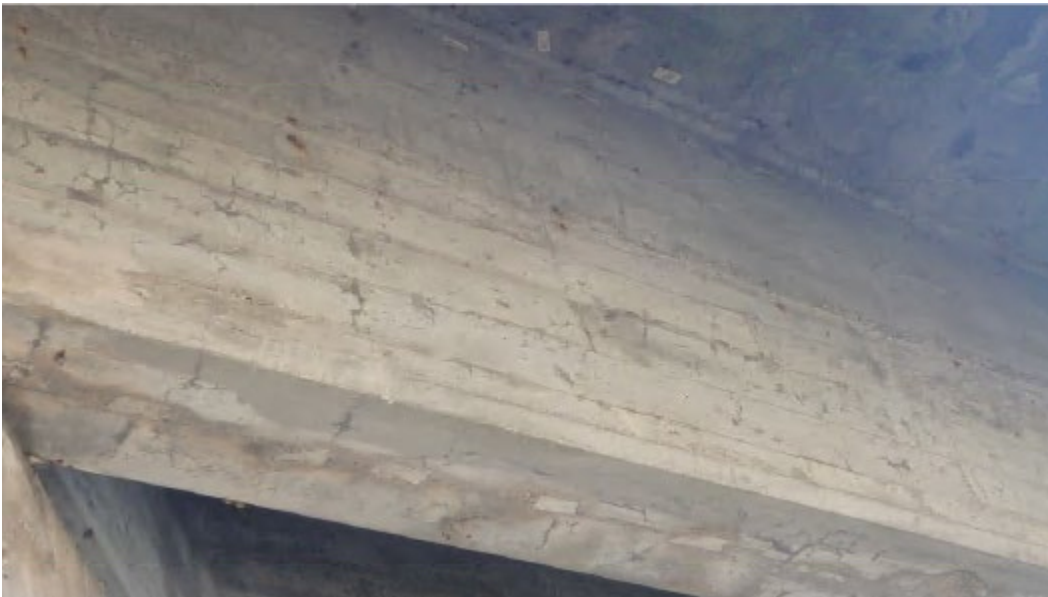
Narrow map cracking
