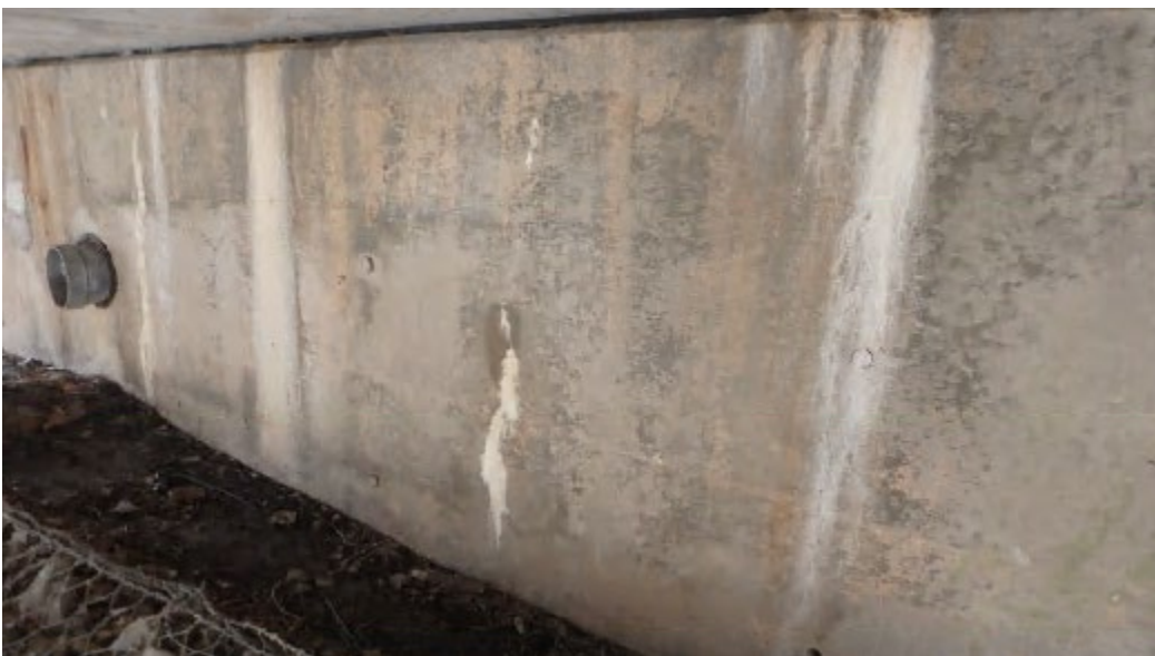
Narrow cracks and drainage blockages
